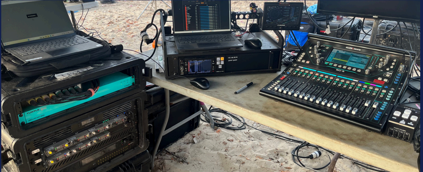
Remote audio control station in Panama featuring the Turtle AV Mineola 8x8, Netgear AV Line switches, and Allen & Heath mixer.
