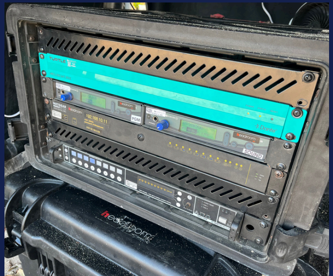
Close-up of the Turtle AV Mineola 8x8 Dante Audio Bridge integrated into the mobile field rack
