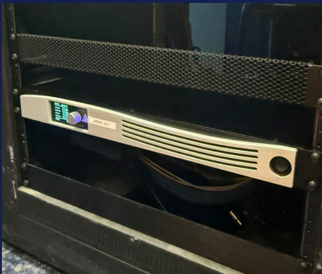
Apex amp in rack. Note the compact size of amp as it occupies the same space in rack as previous unit to drive same speakers.
