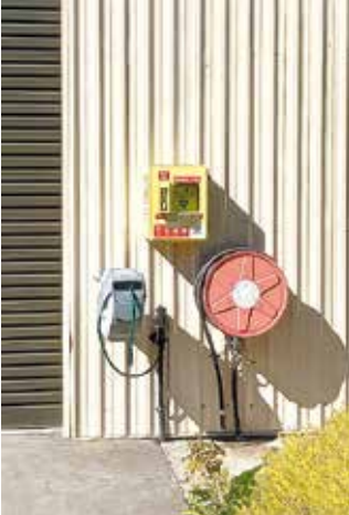
Milnthorpe - 34 Nelson Street: Yellow cabinet on outside wall of shed.
